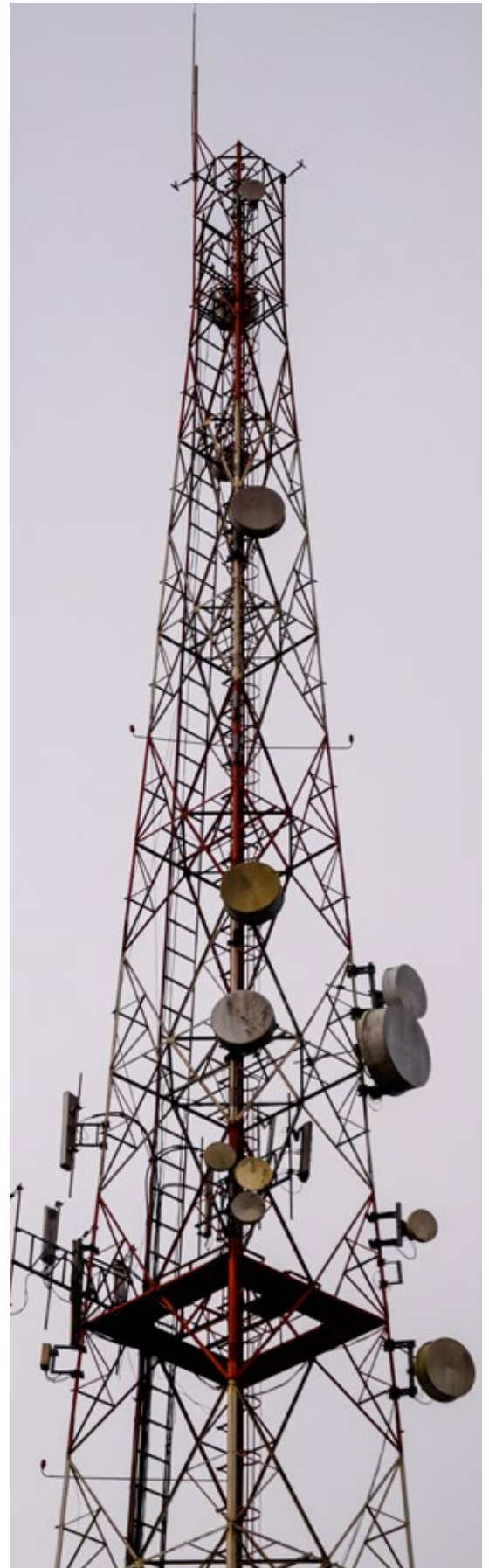
The telecoms sector will change completely with the introduction of 5G
