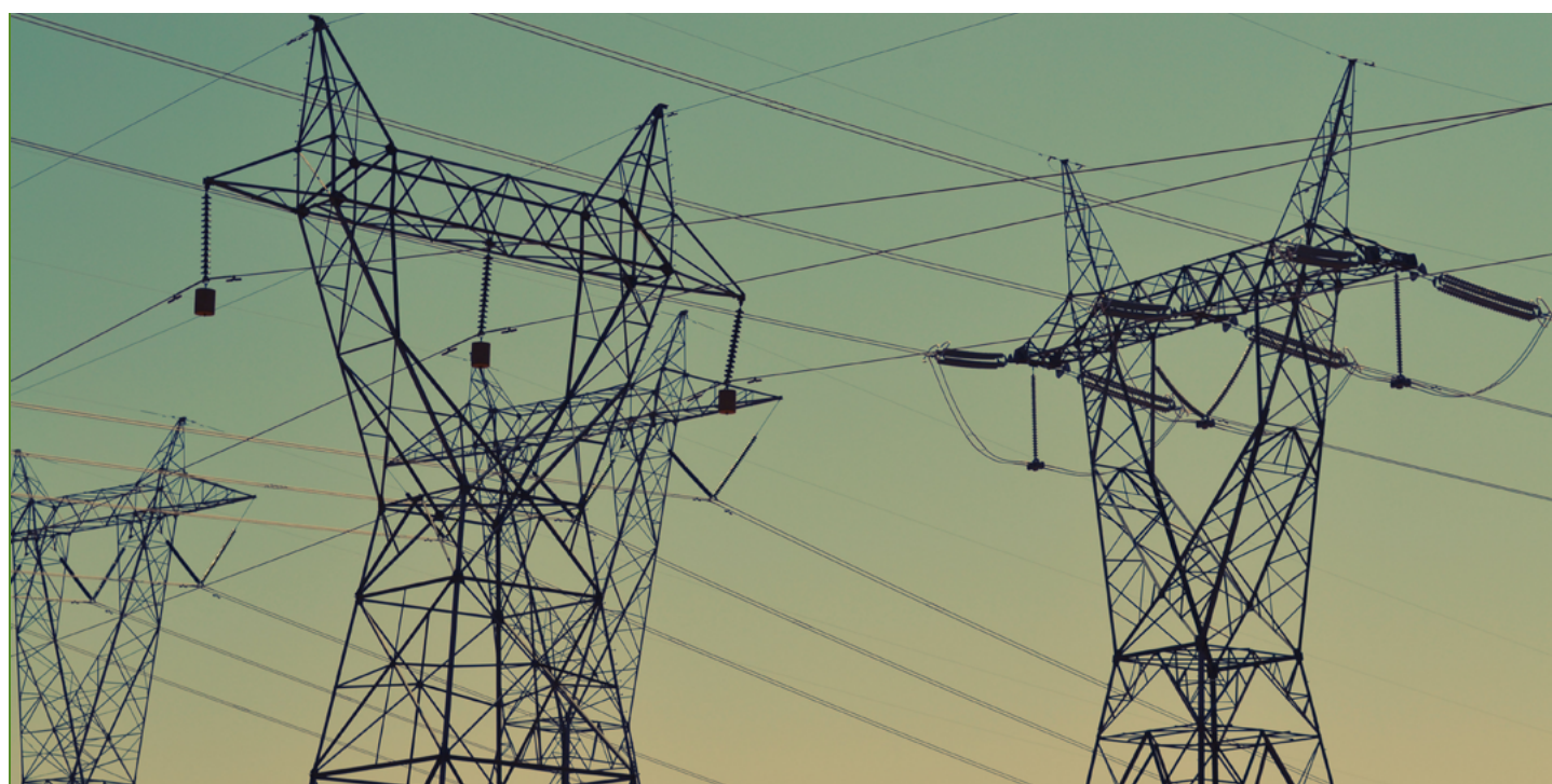
US-based electricity utility company Xcel Energy has committed an undisclosed amount to venture firm Energy Impact Partners' latest fund
